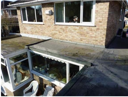
Roof in its original leaking state
